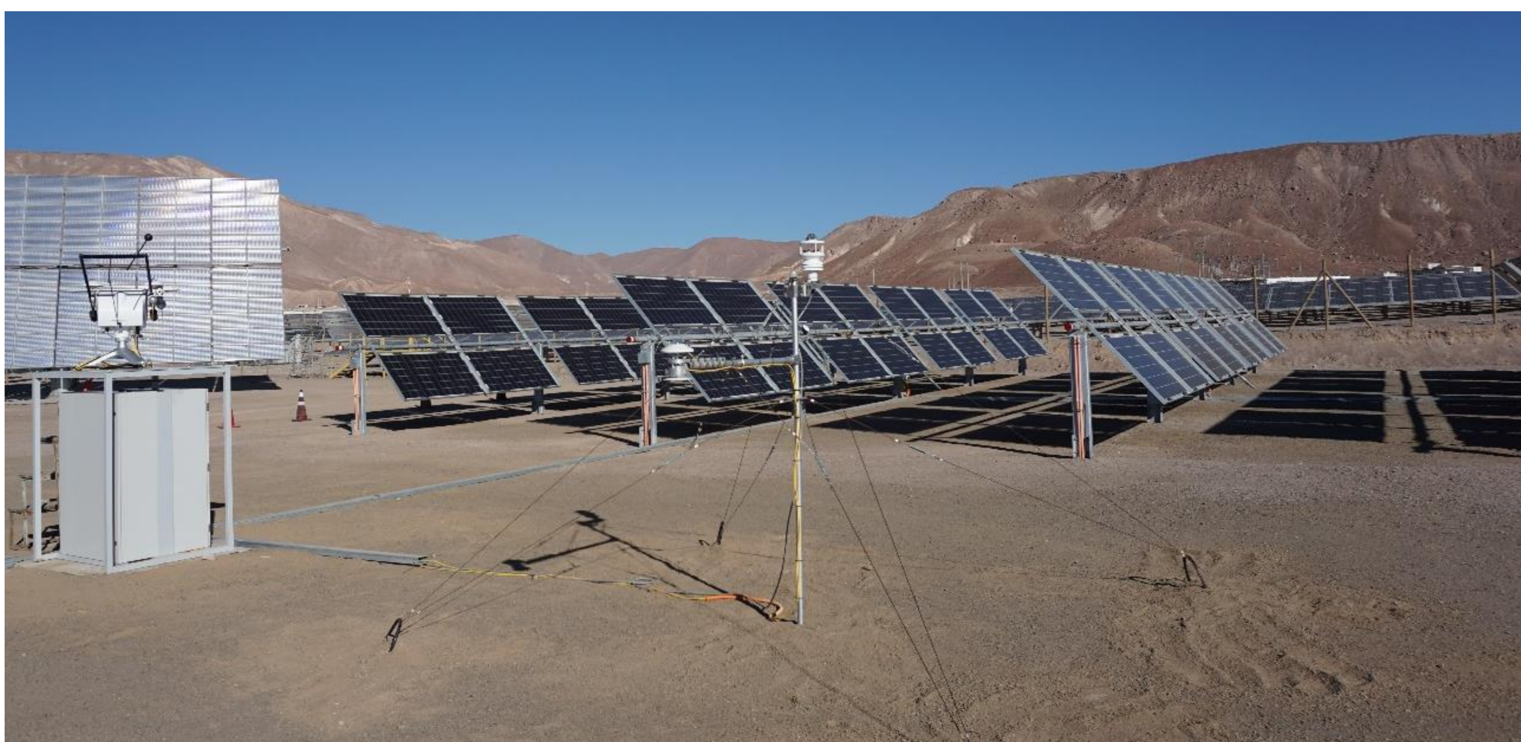
Figure 1 shows a view of the HSAT group of the bifacial pilot as well as the meteo station and albedometer
