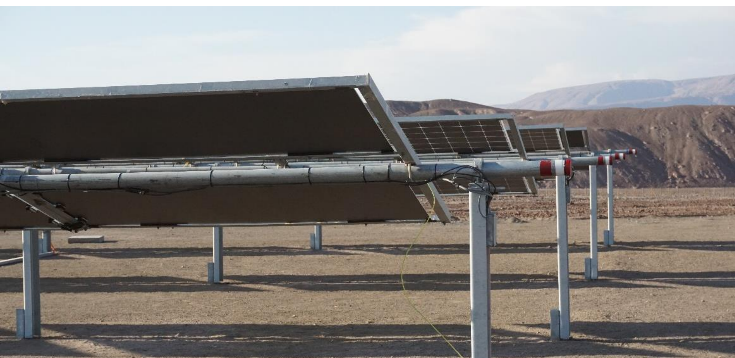
Figure 2 shows a view of the FIX-TILT group. One of each two strings has their rear side covered.
