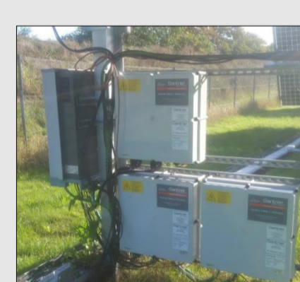
Monitoring independent of inverter measurements
