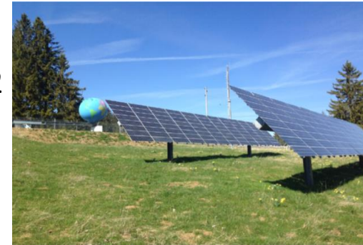
Mont Soleil, Switz. 1992 0.3% annual power loss
