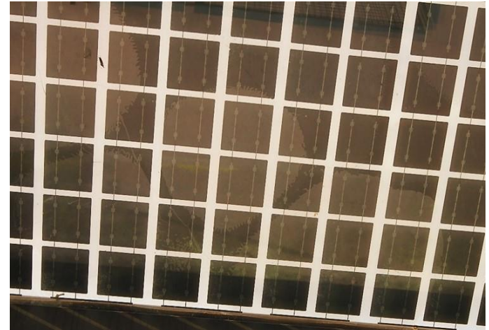
Severe delamination on glass/glass module 10 years, Arizona USA
