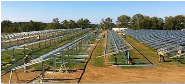
La Hormiga PV Power Plant (commercial), Chile 2
