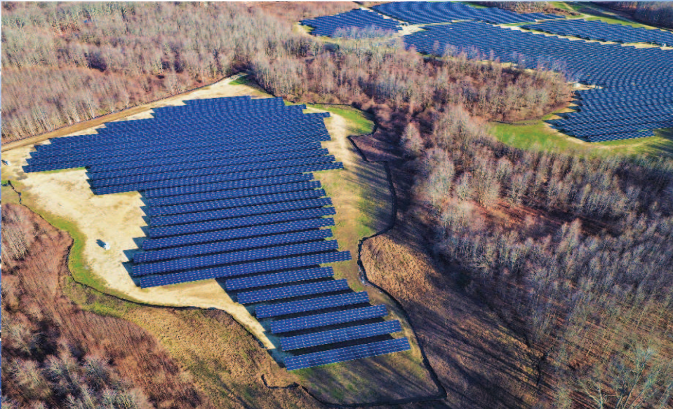
Industrial Power Plant in New Jersey 15MW of Sunpreme Bi-Facial Modules
