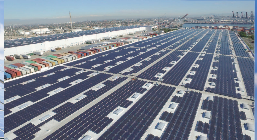
The Largest Commercial Roof-top Installation in the US (Port of Los Angeles) 10MW of Sunpreme Bi-Facial Modules → 15MW
