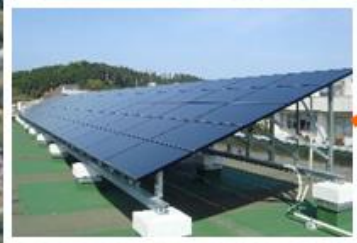
CIGS PV 100 kW Solar Frontier
