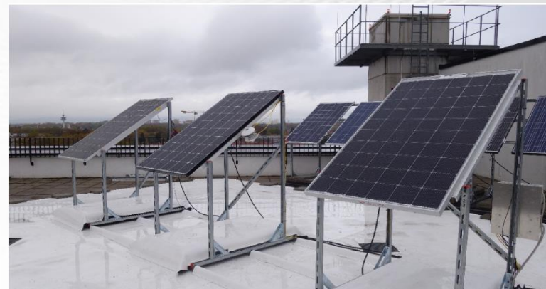
High Albedo(Bright white roofing membrane), Tilt angel 35°
