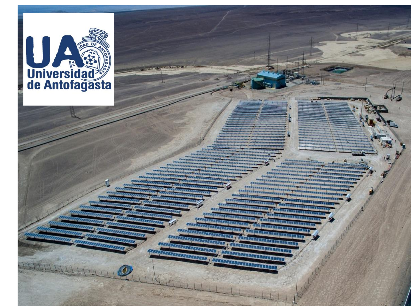
Lalctur Industrial Pilot Plant 1 MW
